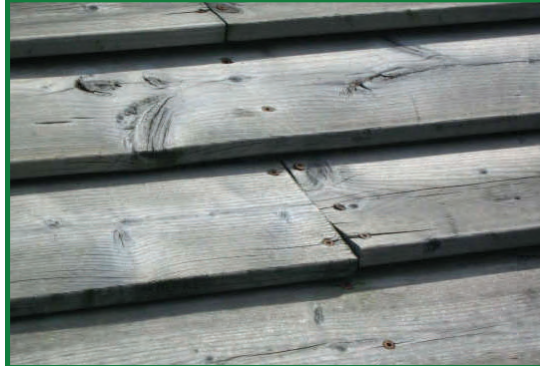
Untreated P.T. fence boards in a 4 y.o. roof:
